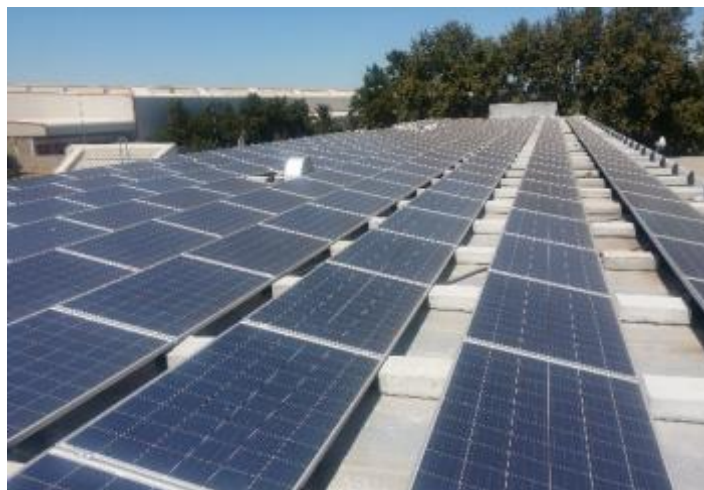
Figure 10. Rooftop Solar PV installation
