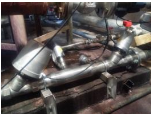
Figure 13. Grey water mixer unit at the dye vessel
