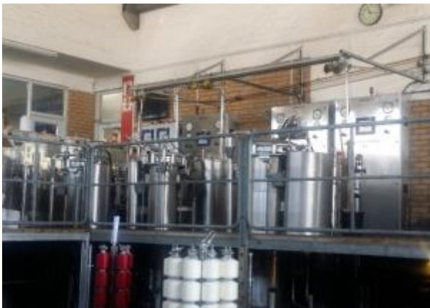
Figure 12. New programmable fill and flush systems installed
