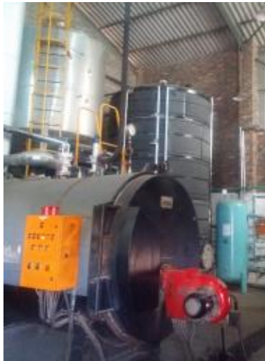
Figure 9. Insulated 60°C tank situated behind the boiler
