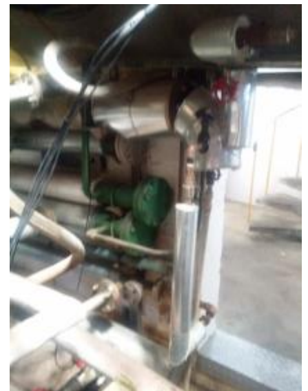
Figure 8. Insulated flanges and piping
