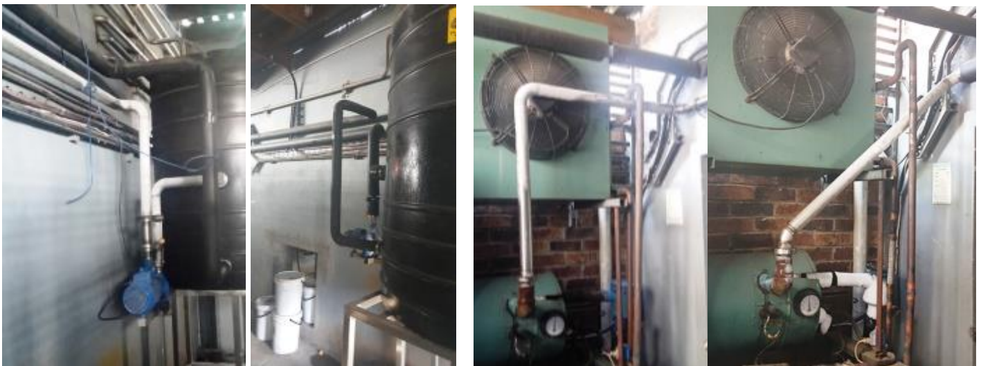
Figure 1. Chilled water piping before and after the insulation and pipe diversion project.
